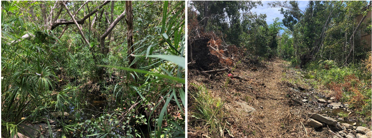
Figure 13. Photos of a gut taken by a resident before (left) and after (right) excavation.
