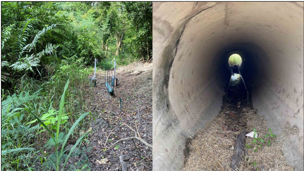
Figure 55. An Onset HOBO U20 Water Level Logger at gauge station SRB01 (left). Water flowing through a concrete structure (right).
