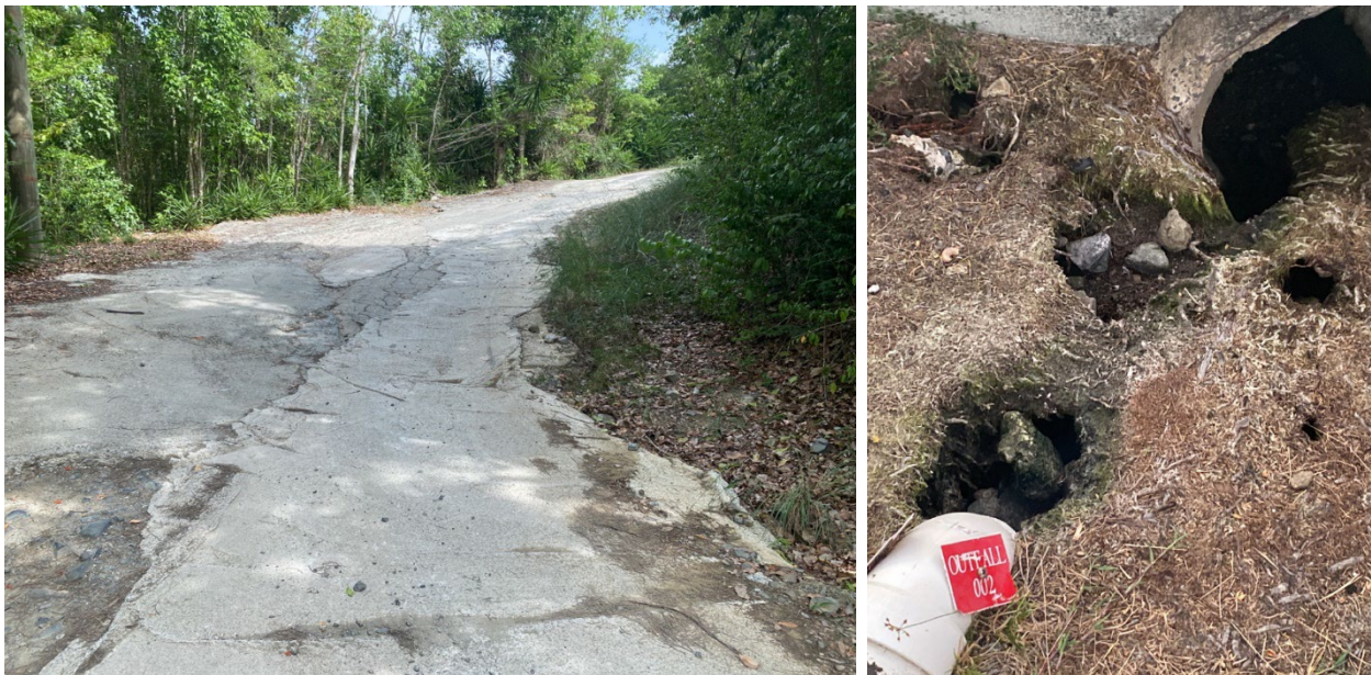
Figure 38. Road erosion (right) and clogged stormwater infrastructure (left).
