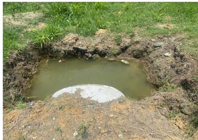
Figure 39. Suspected illicit discharge at an outfall observed during field investigations
