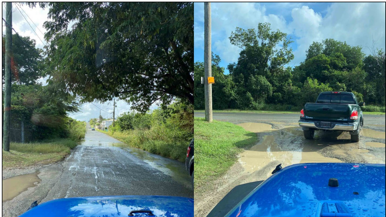
Figure 64. Ponding observed on roads adjacent to the LPB02 and LPB05 monitoring locations after a storm event.
