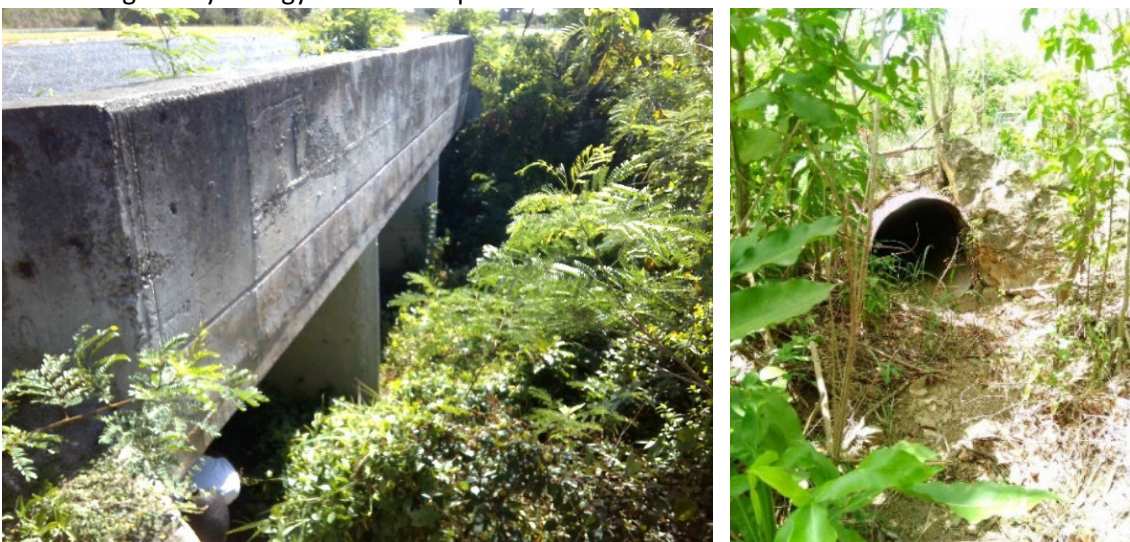
Figure 47. Examples of stormwater infrastructure in the Long Point Bay watershed.
