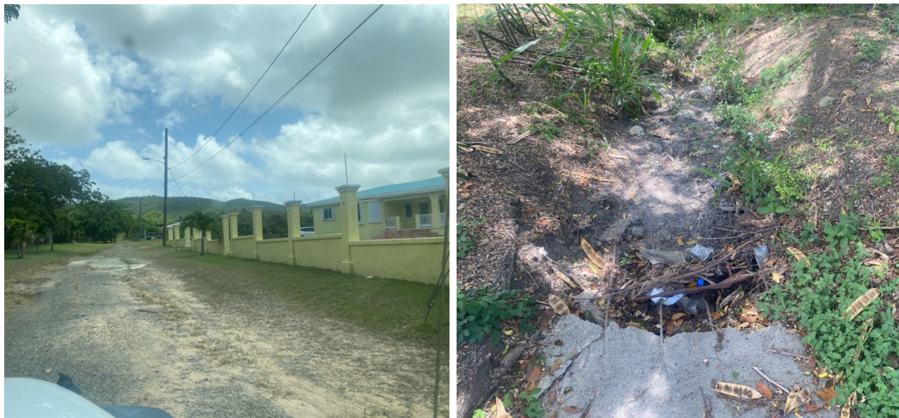
Figure 37. Road erosion (right) and clogged stormwater infrastructure (left).
