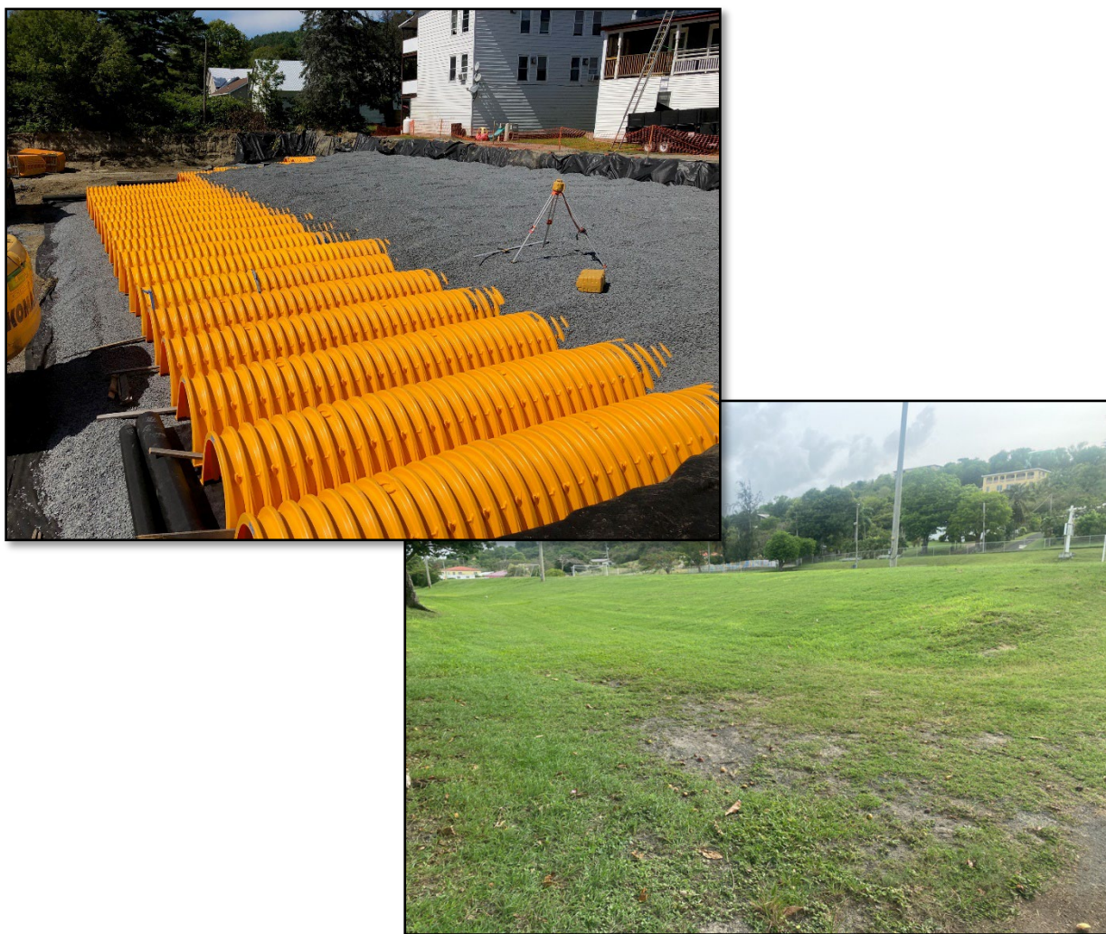
Figure 81. Example photo of subsurface infiltration chambers (above) and recreation field at Freewill Baptist Church (below).
