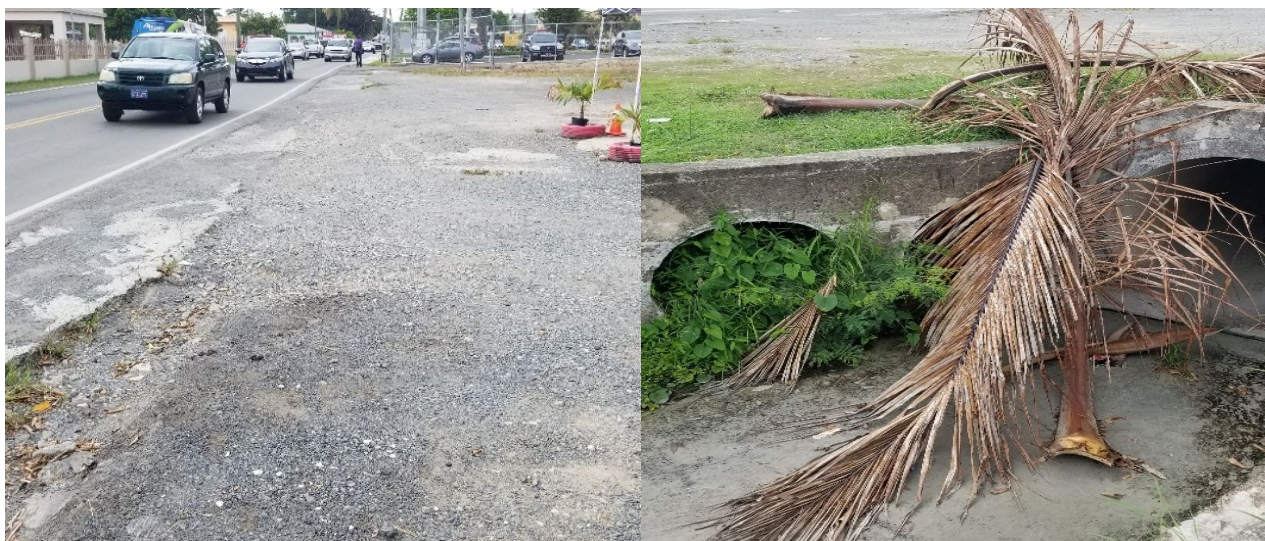
Figure 38. Road erosion (left) and clogged stormwater infrastructure (right).
