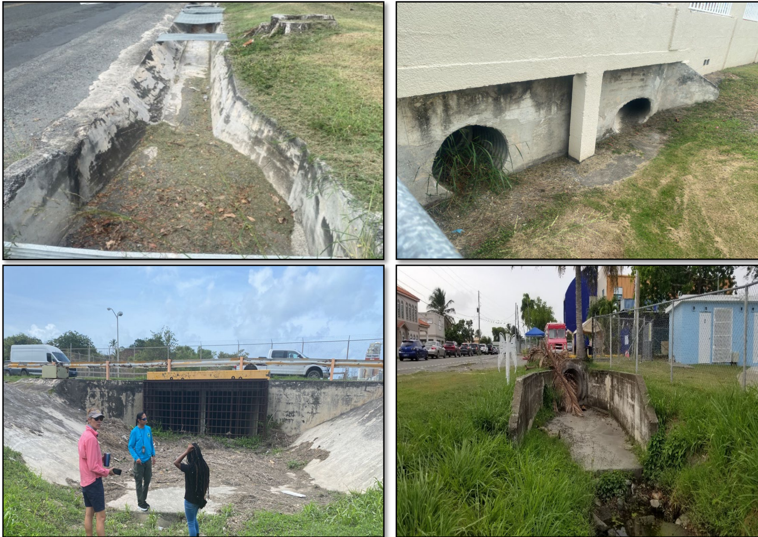
Figure 49. Examples of stormwater infrastructure.
