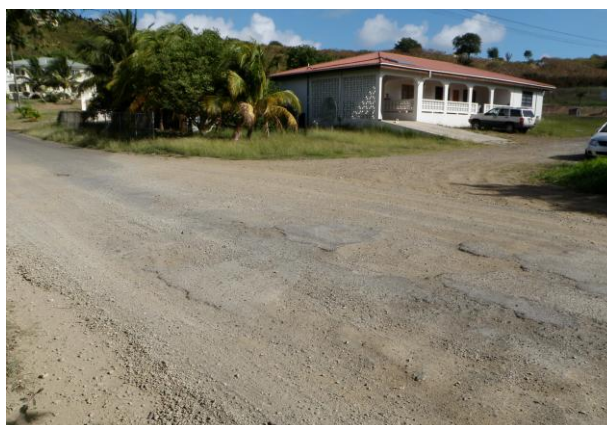
Surface deterioration of South Shore Rd.
