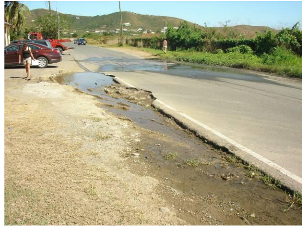
Location at Milgie's where East Gut flow is diverted along the parking area and then across Rt. 624 via an existing paved dip.
