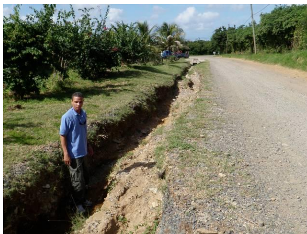
Eroding ditch along lower portion of Seven Flags Rd.
